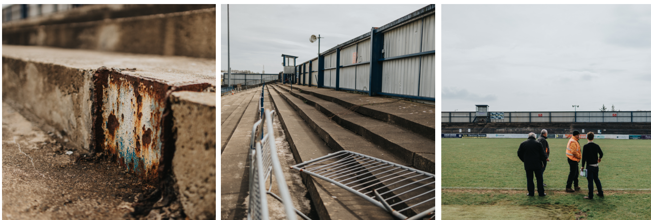
Aging facilities at Coleraine Showgrounds
